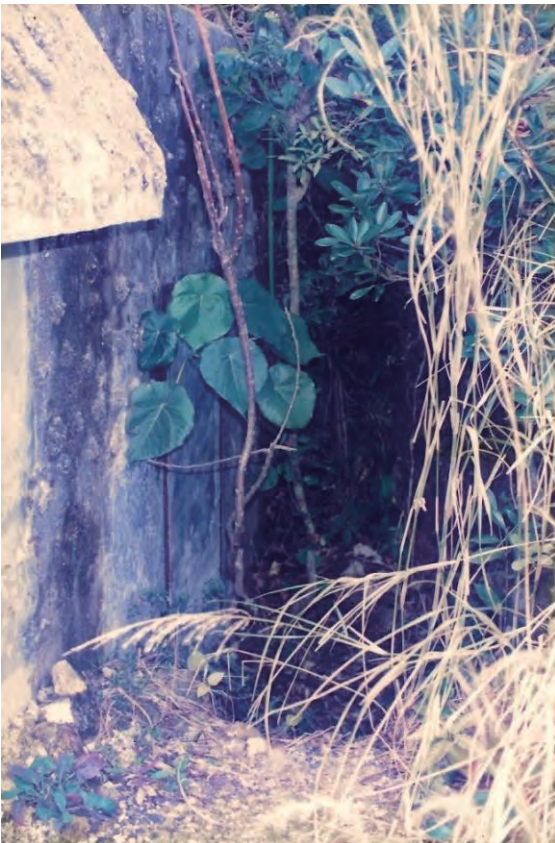
Left side with blocked entry. (February 1997)
