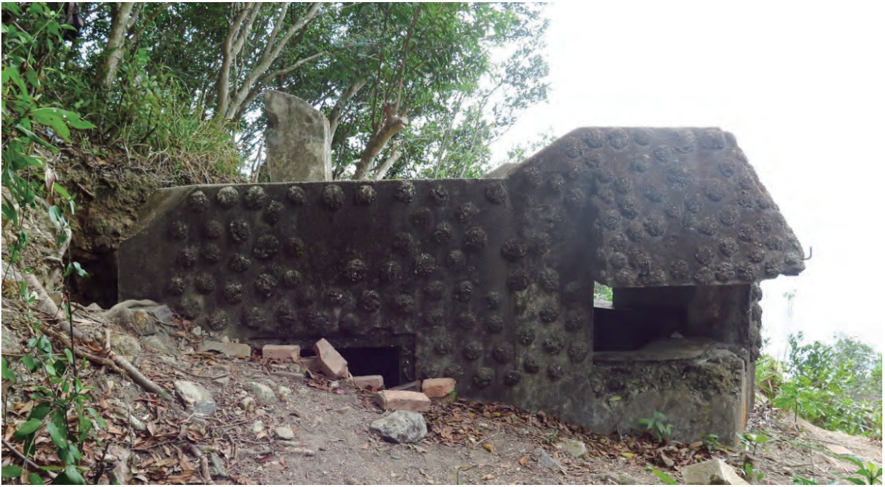
Right side of OP with a blocked entrance. (31 January 2022 by Lawrence W.C. Lai)
