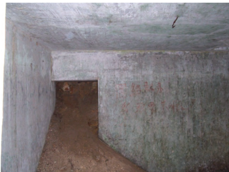
Rear interior wall with the entrance blocked due to radar station construction. (February 1997)
