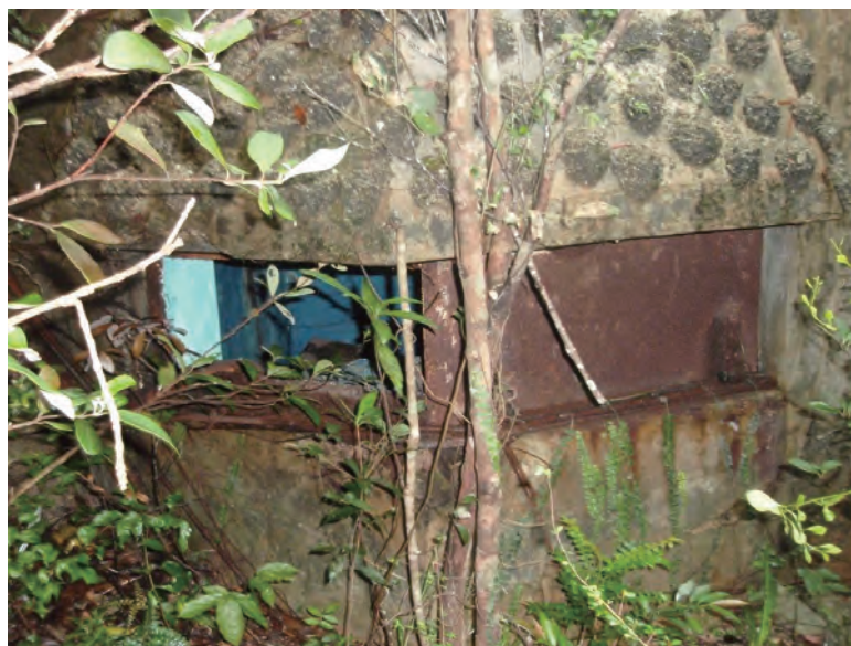
Exterior of loophole, one cover missing. (August 2013)
