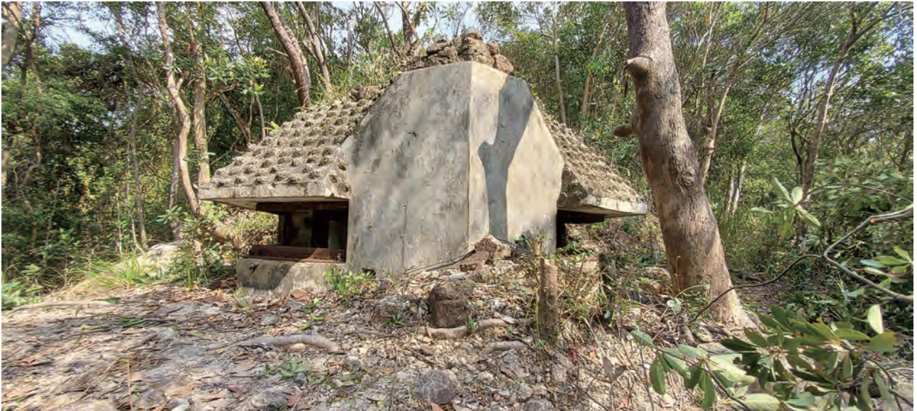
Front view of OP. (7 January 2022 by Lawrence W.C. Lai) Note the rectangular portal for cables close to its right hand aperture near the ground.
