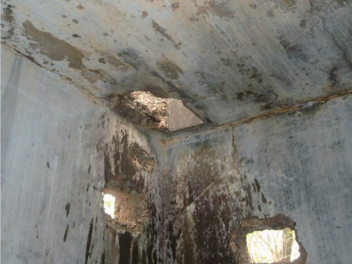
Interior rear right side with two holes cut through walls, and airshaft in roof. (April 2009)
