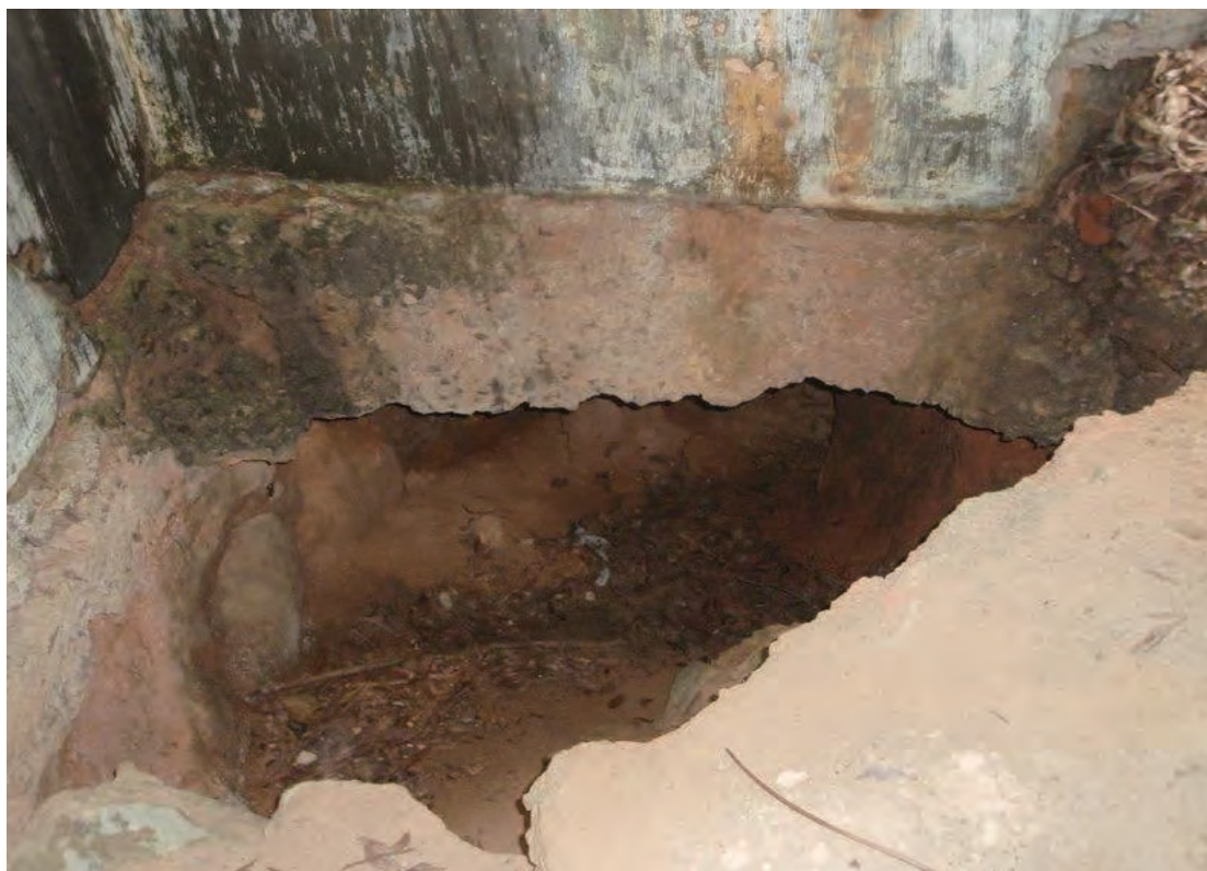
Interior rear with a hole cut through floor for tunnel access. (April 2009)
