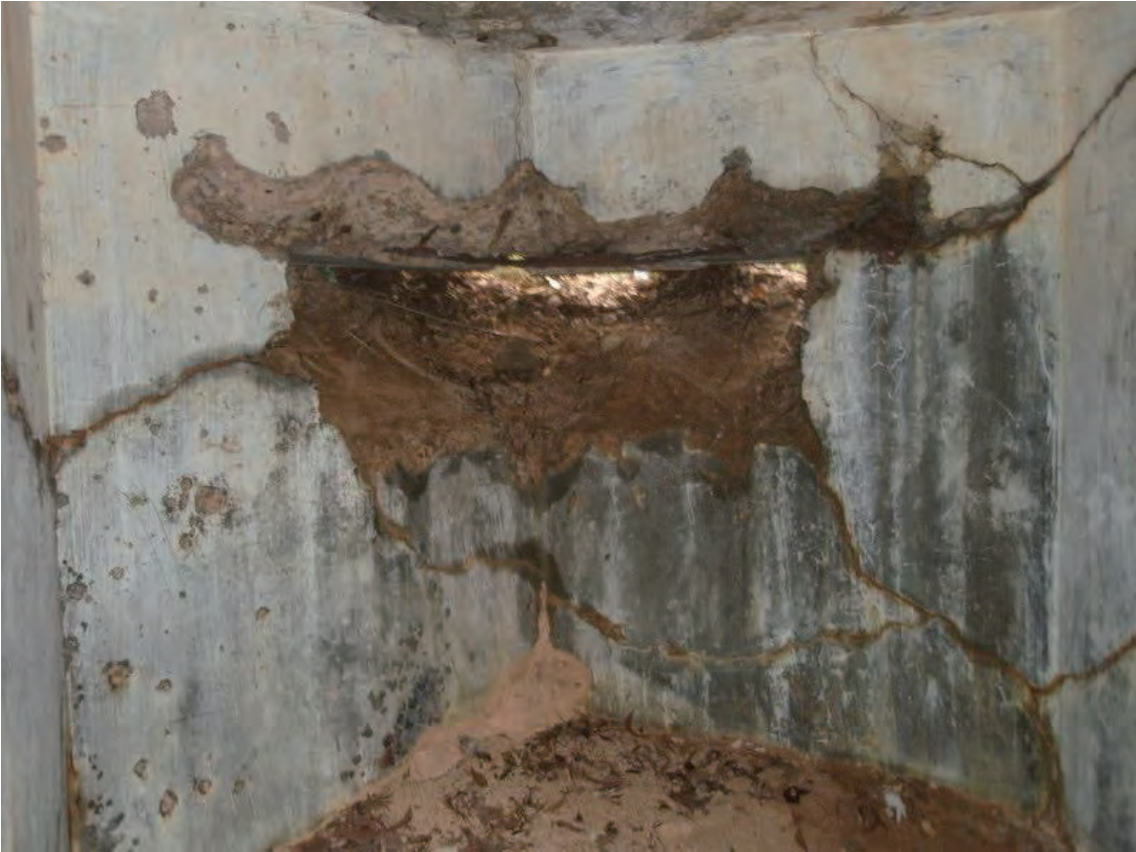
Interior front wall with remains of loophole. Cracks suggest settlement due to loss of ground water and soil erosion due to tunneling. (April 2009)
