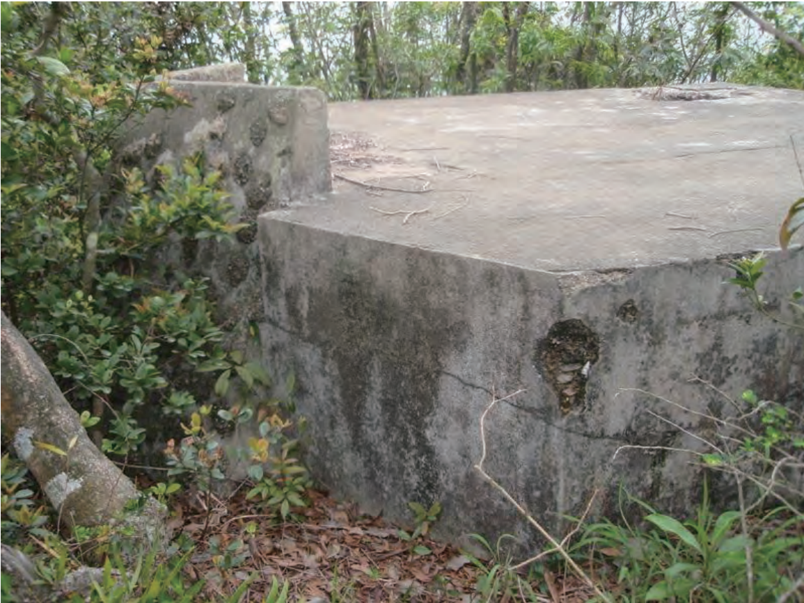
Roof and front left corner. Upper part of air shaft gone. (April 2009)
