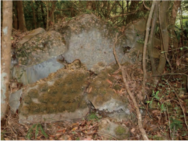
Exterior of ruined front wall. (December 2009)
