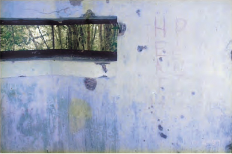
Front right loophole from interior. Note shrapnel damage on wall.
