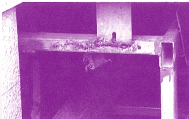
Fig.2 An example of corroded subframe without protection.
