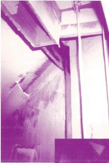
Fig. 3 An example of adverse effects from condensation and moisture attack.
