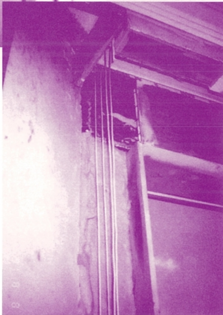
Fig. 4 An example of damaged internal condition of a hotel room.
